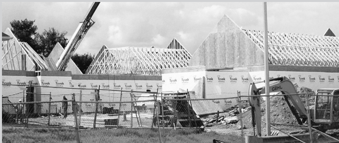
Progress at the new building for MCCH's Adrienne's Safe Havens and offices, and Community Ministries of Rockville's Chase Partnership House.
